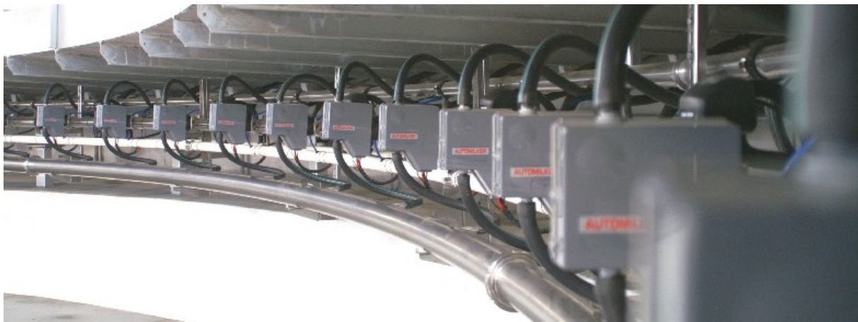
Automilker units installed in a 60 bail rotary dairy installation.
